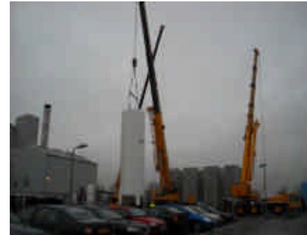
Oxygen Storage Tank
